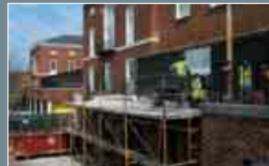
Attendees will learn from the case study of the University of Virginia's Newcomb Hall Student Center renovation project.
